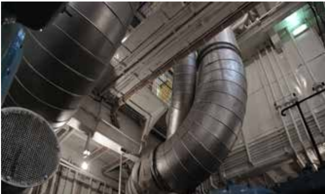
Exhaust gas piping
